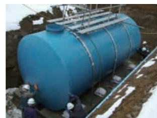
Quake-resistant fire-prevention tank
