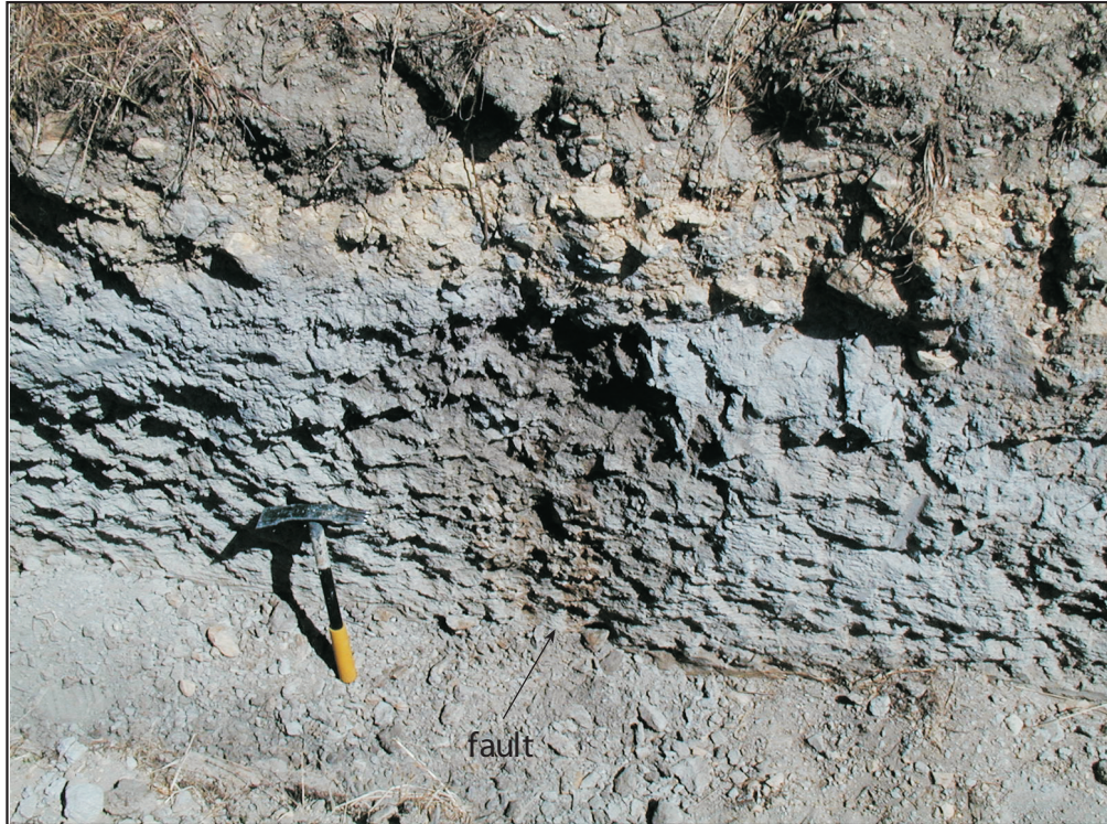
Friable sandstone ( Tof_{b-2a} ) in trench T-1. The friable sandstone generally is weakly bedded and jointed. A small near-vertical fault is indicated by oxidized clay stringers in the sandstone. Photo roll JLB-3.
